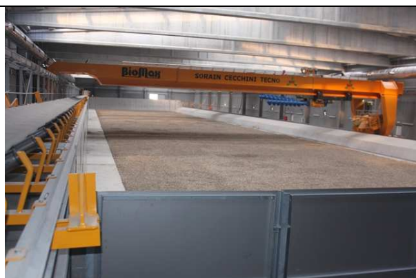
Vista general de reactor
